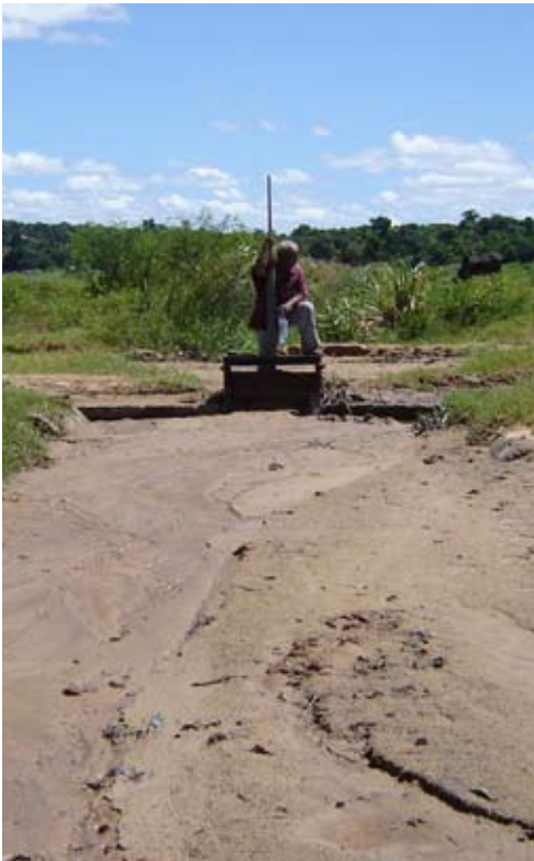
Gap and sand on the main canal called "Karambo" of the check dam of Amboromalandy (Photo : Nosy Alizany, CCAA-Madagascar)
